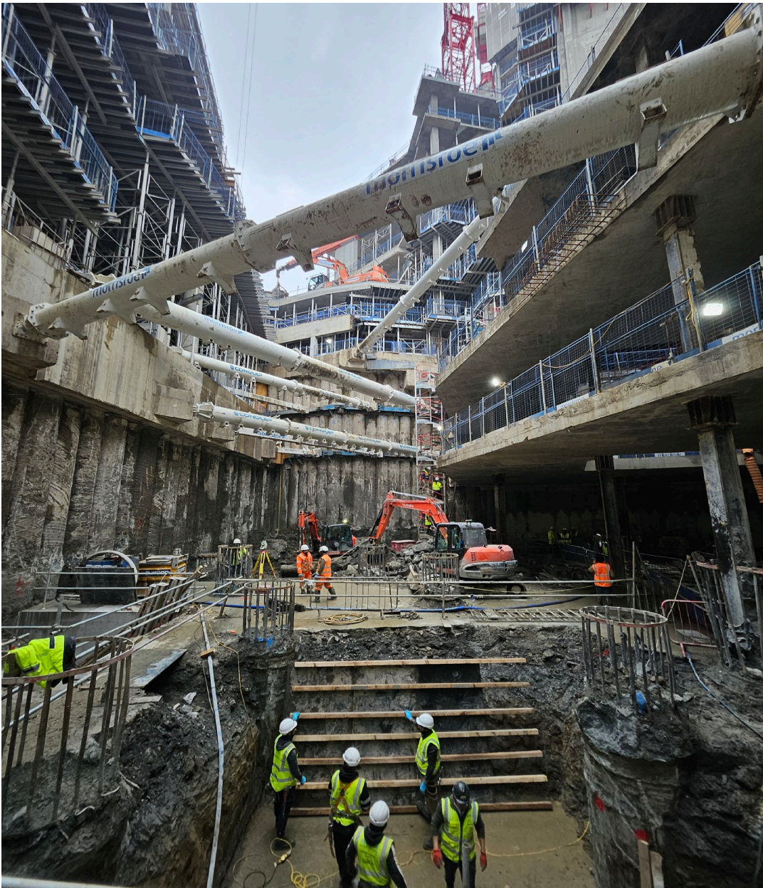
Figure 44: The new station box at Elephant & Castle excavated to its lowest level, 33 metres beneath ground level. Source: TfL
